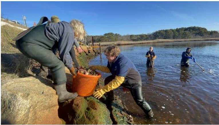
AmeriCorps Cape Cod member Jodi Monroe hands off a basket full of oysters to Wellfleet Assistant Shellfish Constable Johnny 'Clam' Mankevetch on Saturday at the Chequessett Neck dike in Wellfleet. A bed of oysters was moved because of dike construction work. Heather McCarron/Cape Cod Times
