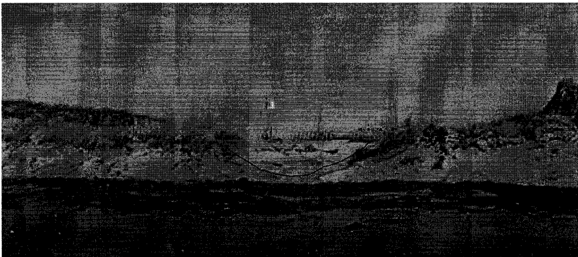
Figure 2.17: Severe erosion, outlined in red (black), which can develop over an established path.
