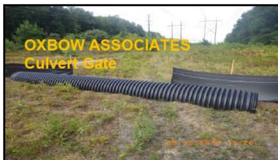
PVC Culvert "Gate"
